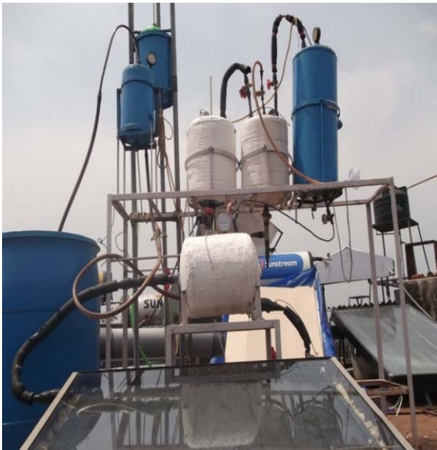
Fig. 3. Photograph of the solar thermal water pump
