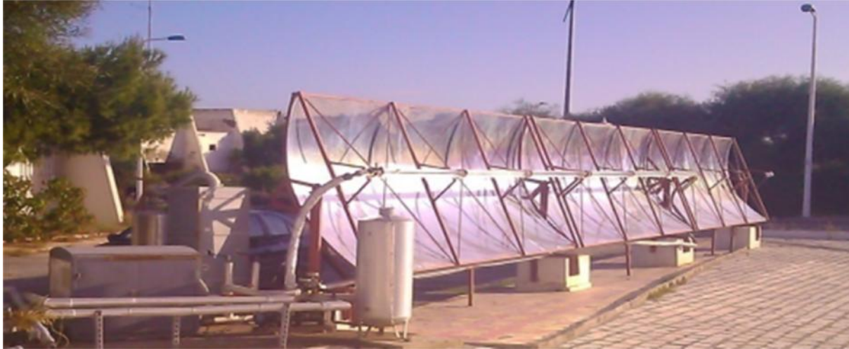
Figure 1: Solar cooling installation
